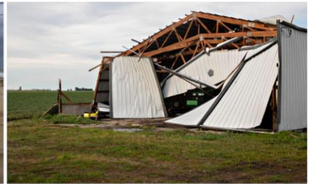
Ciara storm (2020): effects on buildings
